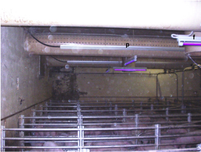
Fig. 2. One of the two units of the trial. The two perforated pipes (p) placed longitudinally in the unit and linked to the corridor of the building provide fresh air; the exhaust air is removed by two fans (f).
